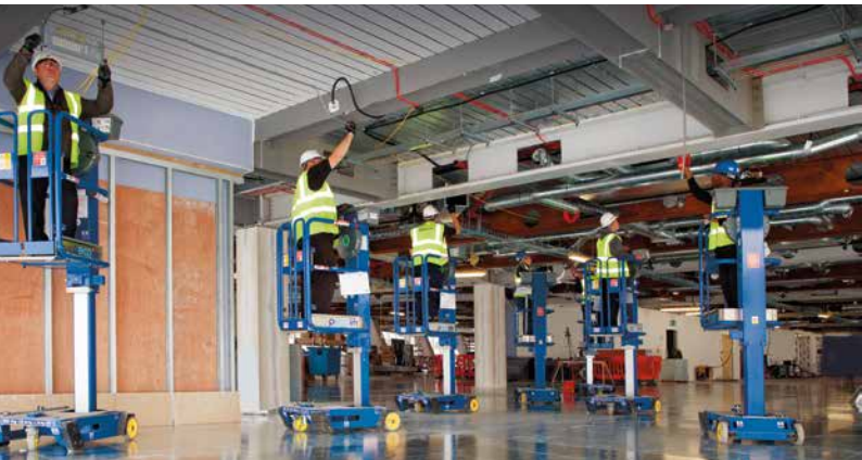
PecoLift in use at the £50m fit-out by ISG plc of the News International Headquarters, London Bridge Place
